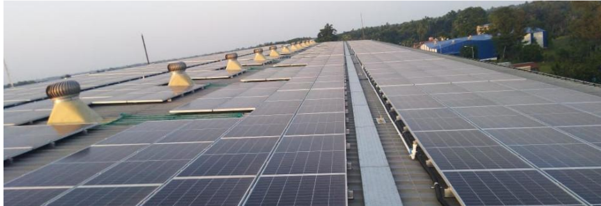
Installed Solar Panels at Amta, Kolkata plant with 531 KW capacity
